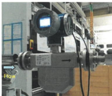
Installation of meter under test (MUT) in calibration line
